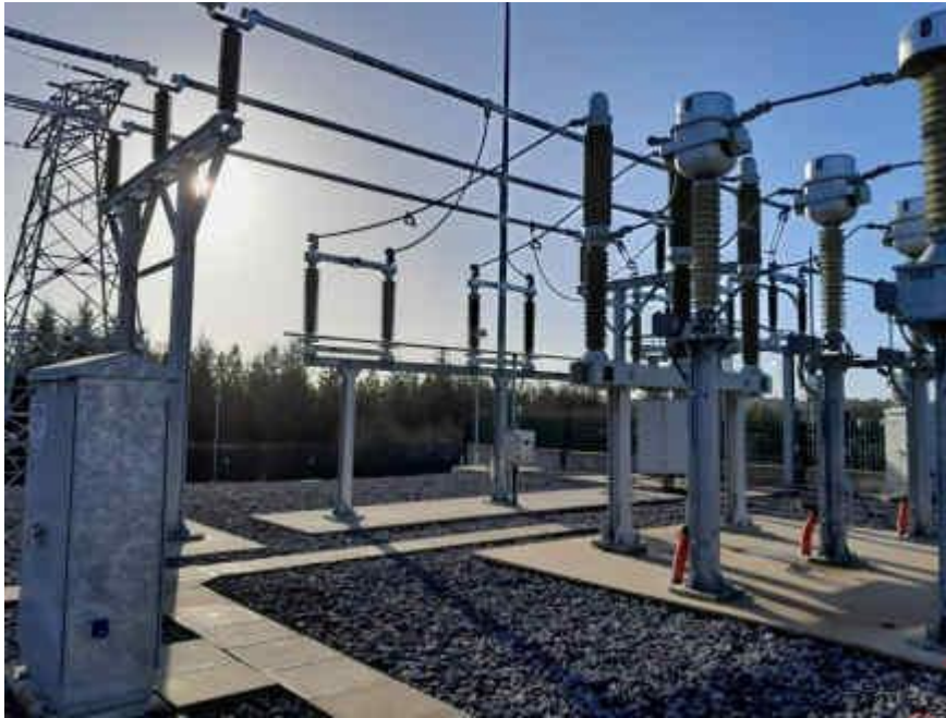
Plate 4-13 Typical 110kV electrical infrastructure
