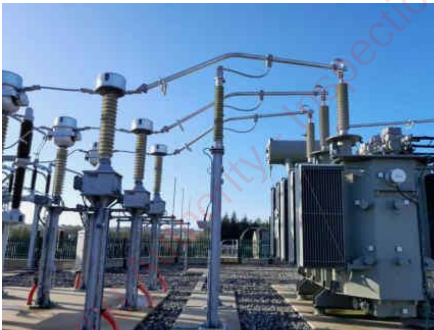
Plate 4-14 Typical 110kV transformer connection
