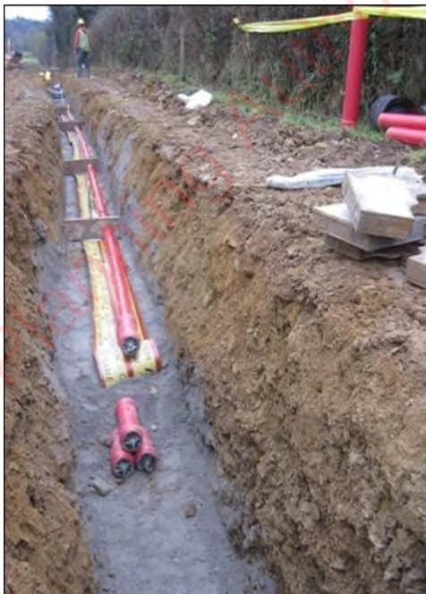
Plate 4-12 Typical Trefoil Cable Trench View
